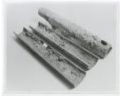
Belmont Lake State Park, Corroded Irrigation Pipes (NYSA_B2877-22_P_B3_F111_002)
