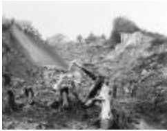
Break in canal at Forestport, N.Y. (NYS A0834-77_B5_F12)
