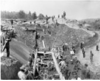
Break in Canal at Forestport, N.Y. (NYS A0834-77_B5_F16)
