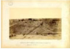
Condition of the work on the new Capitol at Albany, N.Y., photograph D (NYS A1897-78_D)
