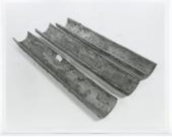
Belmont Lake State Park, Corroded Irrigation Pipes (NYSA_B2877- 22_P_B3_F111_003)
