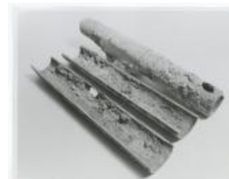
Belmont Lake State Park, Corroded Irrigation Pipes (NYSA_B2877-22_P_B3_F111_002)
